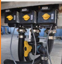
3 electric valves for 3 lane application.
